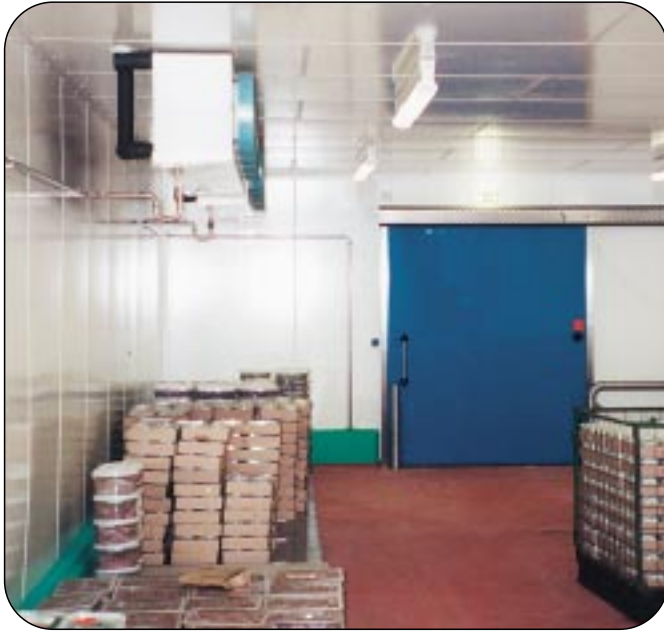
Cold storage room for delicatessen. Totally equipped with GRP- Insulating Panels by ECP.
